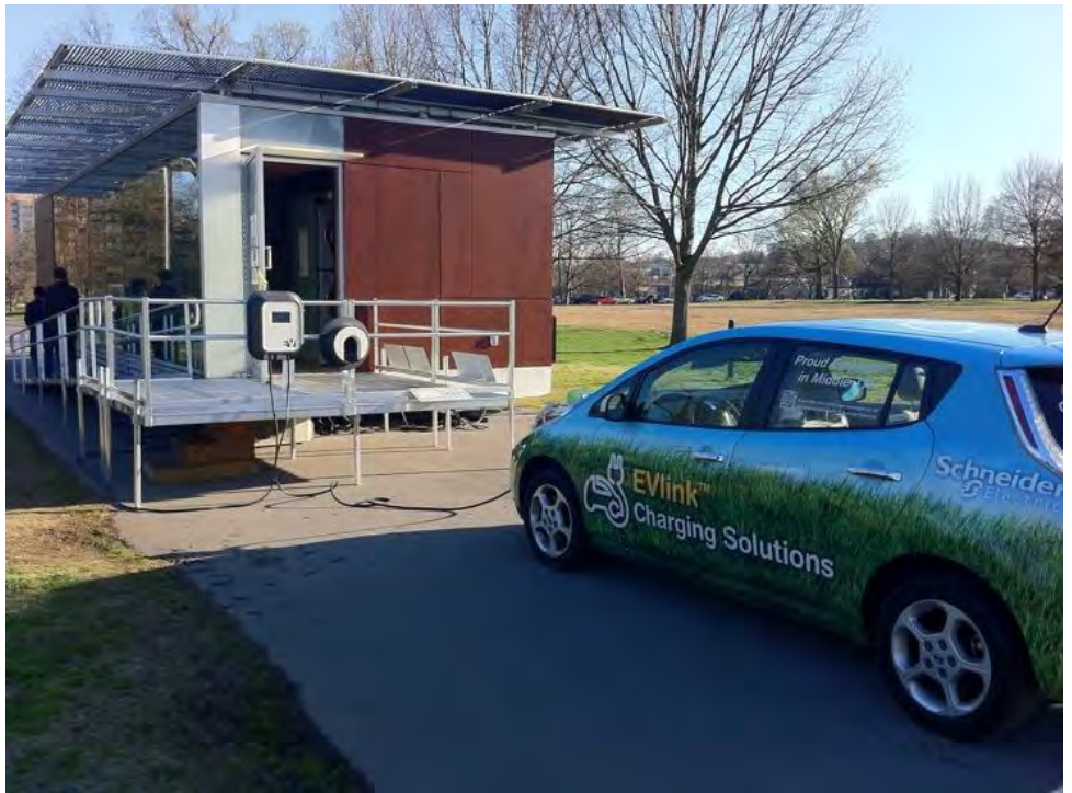
Electric car charging station
