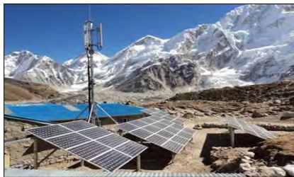
Power for Cellular Towers
