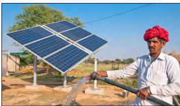
Village Water Pumping
