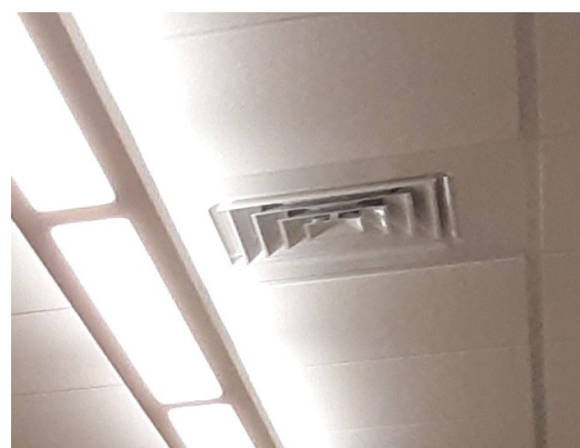
Figure 1. Typical outside supply air diffuser found in a laboratory HVAC system. (Image courtesy of CCS.)
