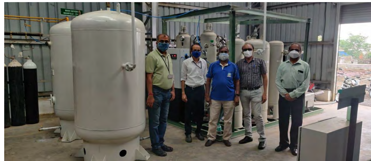
Successfully Commissioned at Aundh Chest Hospital, Pune Coupled to Liquid O 2 plant and GO 2 Plant
