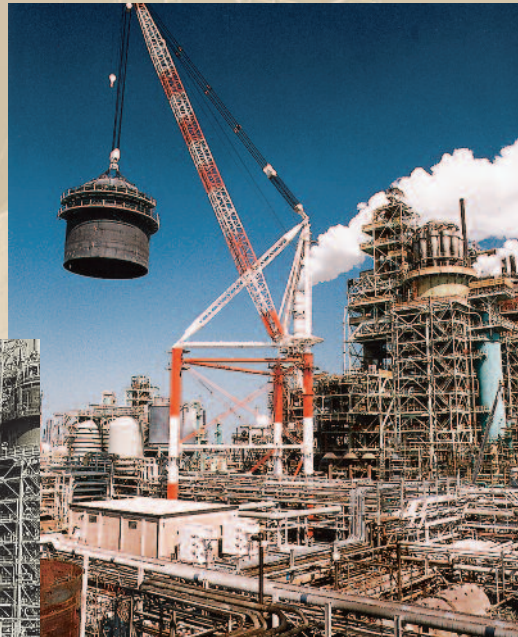
PCLA #1, and #3 are shown in the 1946 photograph on the left. PCLA #1 was dismantled in 1963. The spot where it stood is to the left of the crane in the 1995 photograph (right) made during the replacement of PCLA #3’s regenerator.
