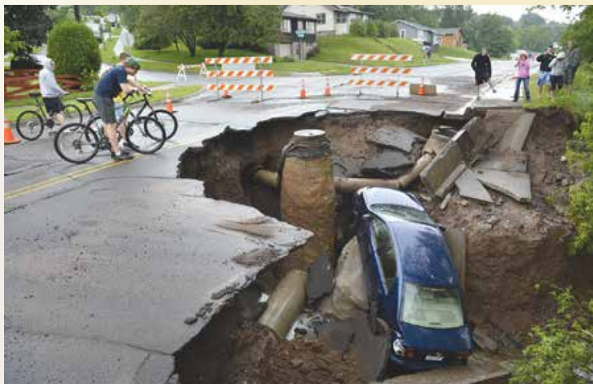
A sinkhole opened in Duluth, Minn., on June 20, 2011. Steady torrential downpours caused residents to evacuate their homes and this car to fall into the sinkhole.
