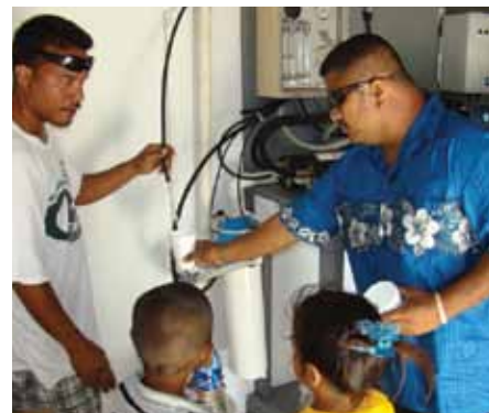
Utrik local government technician Beasa Beasa (above right) uses a solar-powered device that dispenses fresh, clean drinking water.
