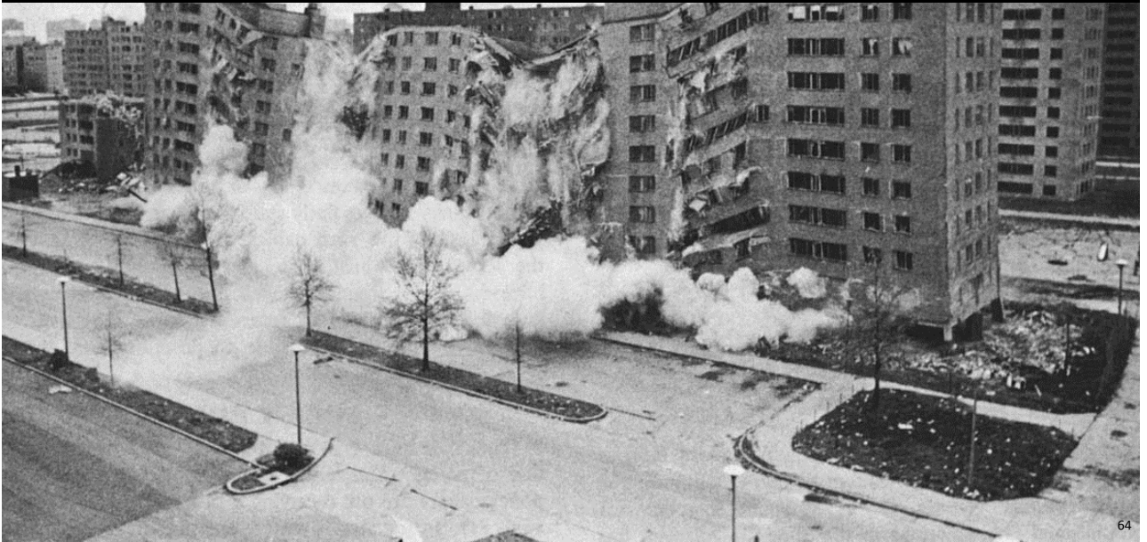
Demolition of Pruitt-Igoe signalled the beginning of postmodernism 1971-72, St. Louis, Missouri, USA
